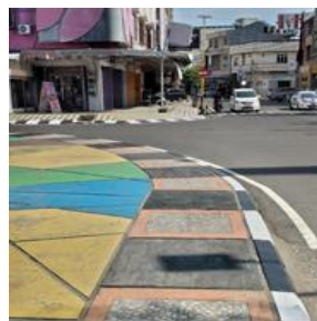
Figure 7. Road Deviation: Ramp And Signs Are Missing
