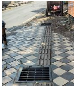
Figure 5. Sidewalk Obstacles: Potholes and Trash Bins
