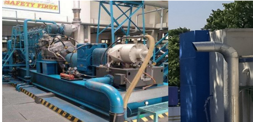
Figure 1. Medium Diesel engine and its exhaust pipe
